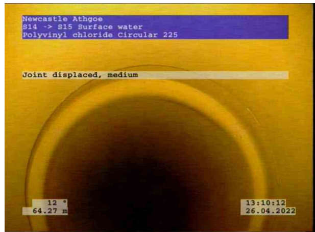
8, 00:05:55, 64.27 m Joint displaced, medium
