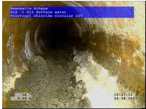
2, 00:00:08, 0.00 m Settled deposits, fine, 5% cross-sectional area loss
