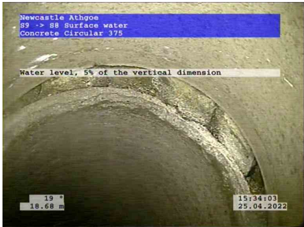
13, 00:02:48, 18.68 m Joint displaced, large
