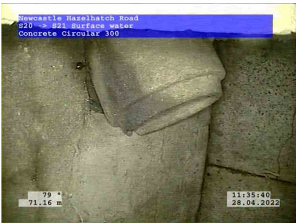
7, 00:06:21, 71.19 m Finish node, manhole, reference: S21, BURIED. NO COVER. GULLY CONNECTED
