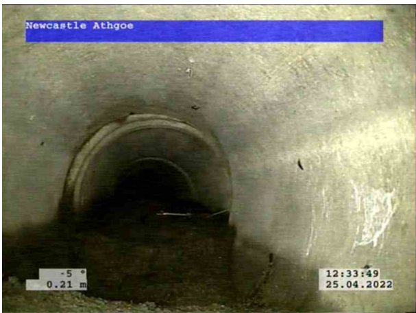
3, 00:00:49, 0.21 m Survey abandoned, UNABLE TO SURVEY. ECXTENSIVE JETTING REQUIRED
