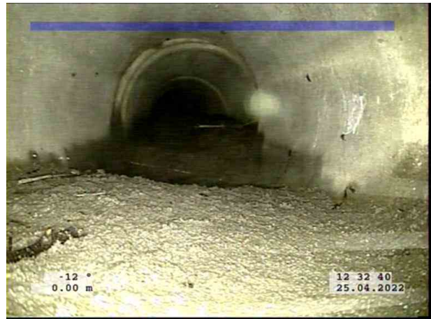
2, 00:00:08, 0.00 m Settled deposits, fine, 25% cross-sectional area loss, start
