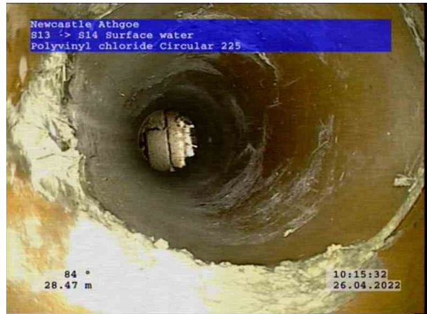
2, 00:01:55, 28.47 m Connection other than junction at 10 o'clock, 150mm dia
