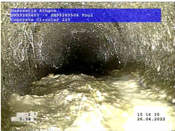
3, 00:01:10, 5.34 m Attached deposits, fouling from 5 o'clock to 7 o'clock, 10% cross-sectional area loss
