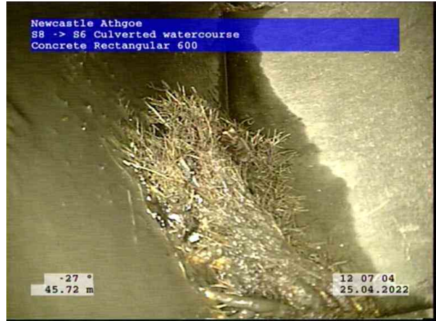
14, 00:06:47, 45.72 m Roots, fine at joint
