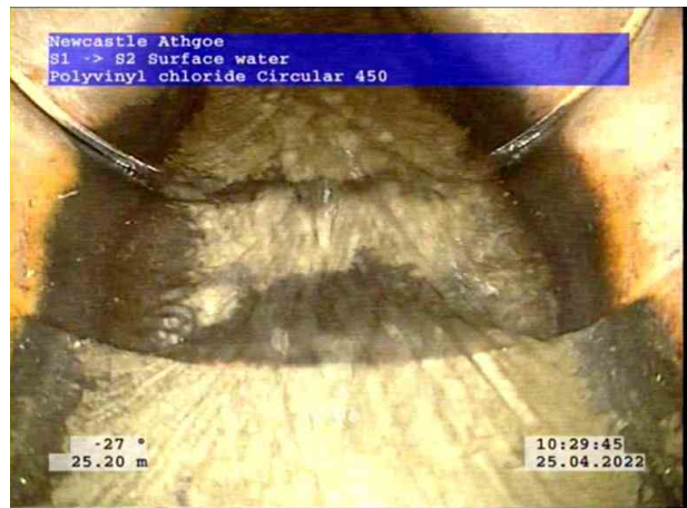
4, 00:03:05, 25.20 m Open joint, large
