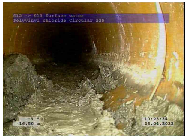
4, 00:02:10, 16.50 m Survey abandoned, UNABLE TO SURVEY. JETTING REQUIRED.
