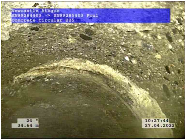
5, 00:03:46, 34.64 m Attached deposits, encrustation from 12 o'clock to 5 o'clock, 5% cross-sectional area loss
