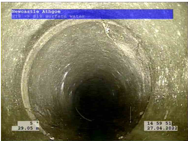
15, 00:03:16, 29.05 m Joint displaced, medium
