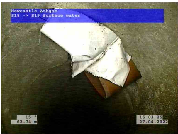
19, 00:06:20, 62.74 m Connection defective, connecting pipe is intruding at 2 o'clock, 150mm dia, intrusion: 20%
