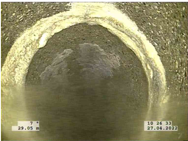
3, 00:02:54, 29.05 m Attached deposits, encrustation at joint from 12 o'clock to 12 o'clock, 10% cross-sectional area loss
