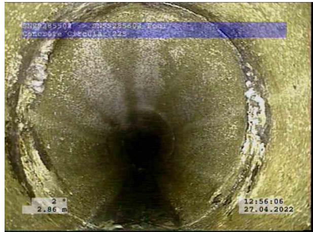
2, 00:00:29, 2.86 m Attached deposits, encrustation at joint from 12 o'clock to 12 o'clock, 5% cross-sectional area loss
