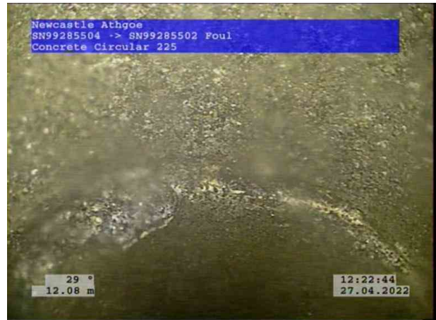
2, 00:01:24, 12.08 m Attached deposits, encrustation at joint from 7 o'clock to 11 o'clock, 5% cross-sectional area loss
