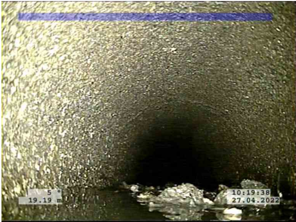
5, 00:02:37, 19.19 m Settled deposits, fine, 30% cross-sectional area loss
