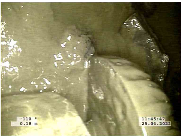
3, 00:01:00, 0.18 m Settled deposits, fine, 15% cross-sectional area loss
