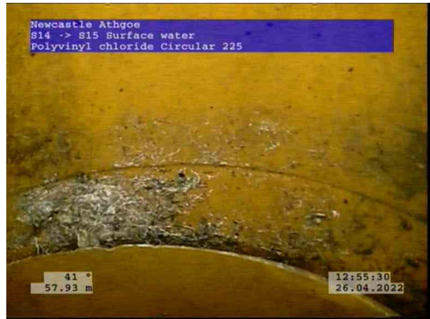
6, 00:04:31, 57.93 m Open joint, large
