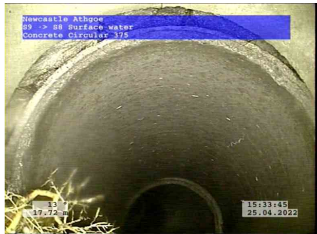
12, 00:02:36, 17.72 m Joint displaced, large
