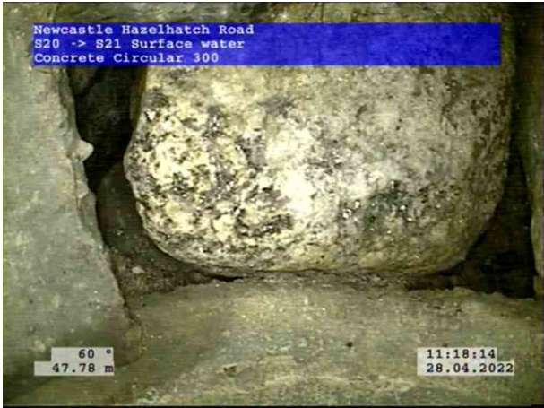
5, 00:03:57, 47.78 m Hole in drain or sewer from 11 o'clock to 1 o'clock
