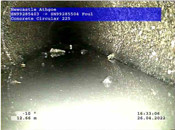
5, 00:03:09, 12.66 m Survey abandoned, unable to survey. extensive jetting required
