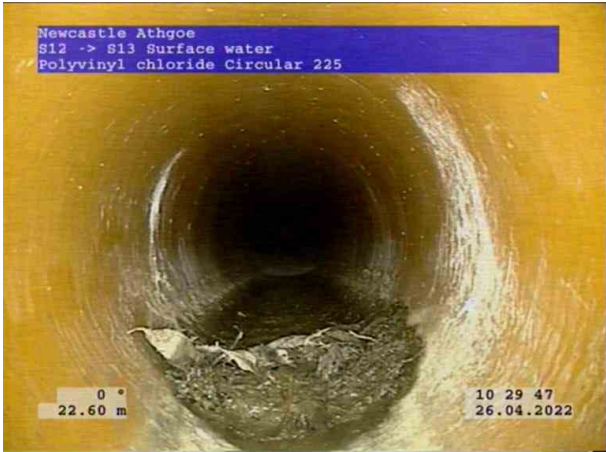
5, 00:02:17, 22.60 m Settled deposits, fine, 5% cross-sectional area loss
