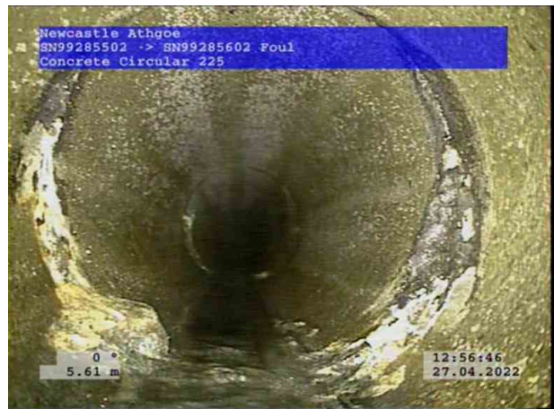
4, 00:00:55, 5.61 m Attached deposits, encrustation at joint from 4 o'clock to 8 o'clock, 10% cross-sectional area loss
