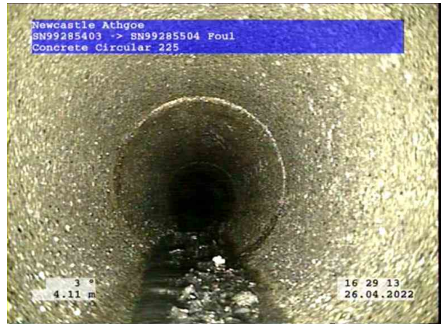
2, 00:00:32, 4.11 m Ingress of gravel from 5 o'clock to 7 o'clock, 5% cross-sectional area loss, start
