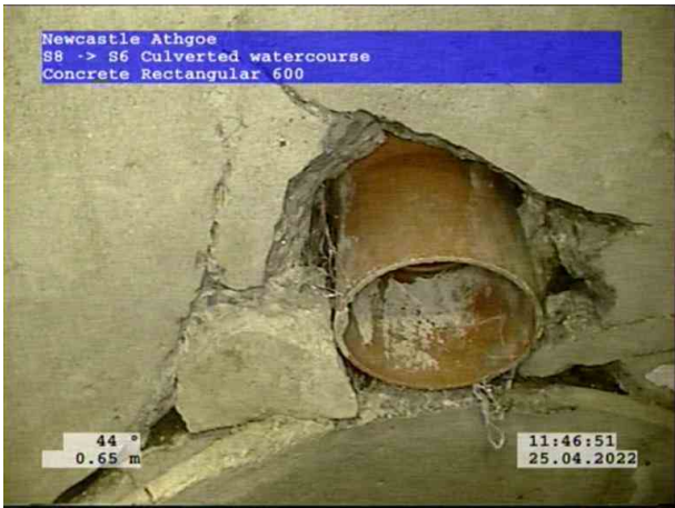
5, 00:01:18, 0.65 m Connection other than junction at 12 o'clock, 150mm dia
