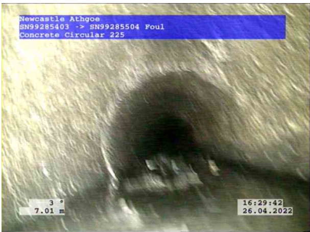
3, 00:01:21, 8.24 m Settled deposits, fine, 15% cross-sectional area loss
