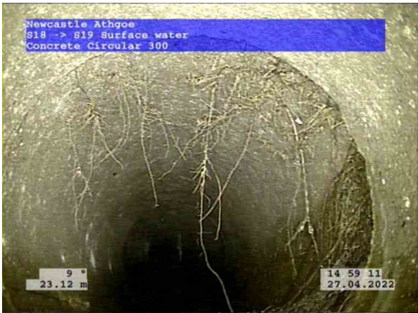
13, 00:02:42, 23.12 m Roots, fine at joint
