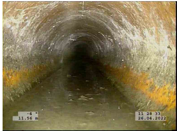
6, 00:05:00, 11.56 m Settled deposits, fine, 10% cross-sectional area loss, start
