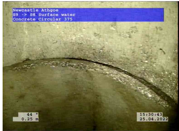
2, 00:00:16, 0.25 m Joint displaced, medium
