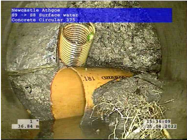
17, 00:04:30, 36.84 m Connection other than junction at 4 o'clock, 150mm dia
