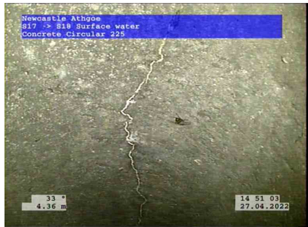
4, 00:00:31, 4.36 m Crack, longitudinal at 1 o'clock
