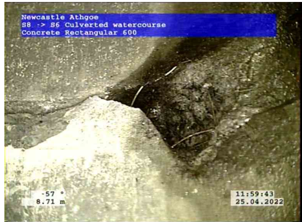
2, 00:00:43, 8.71 m Hole in drain or sewer at 7 o'clock
