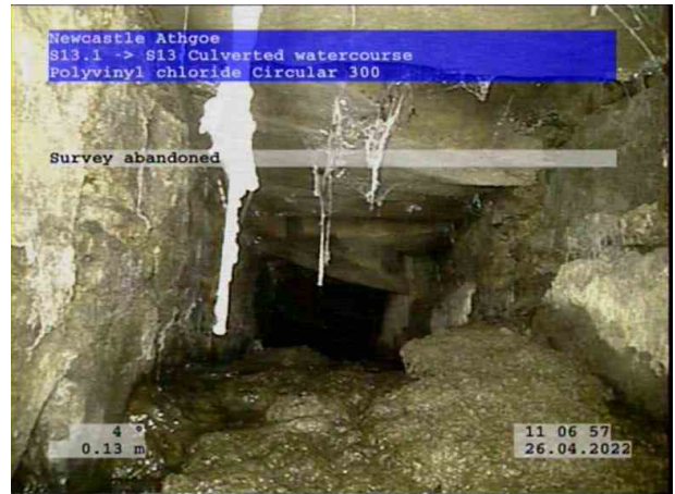
2, 00:00:31, 0.13 m Survey abandoned, UNABLE TO SURVEY. CULVERT
