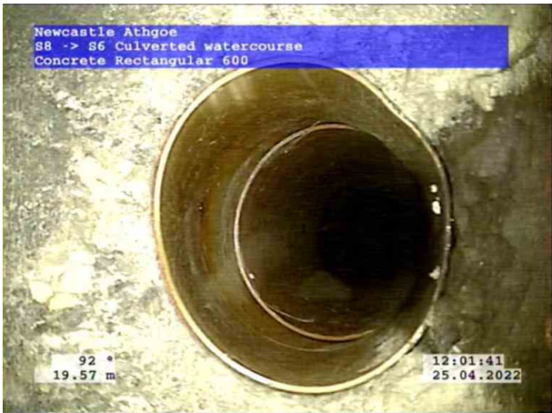
5, 00:02:24, 19.57 m Connection other than junction at 3 o'clock, 150mm dia
