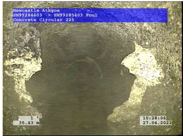
6, 00:03:56, 35.43 m Attached deposits, encrustation at joint from 3 o'clock to 9 o'clock, 15% cross-sectional area loss
