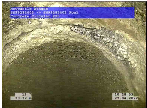
8, 00:04:25, 38.32 m Attached deposits, encrustation at joint from 12 o'clock to 6 o'clock, 5% cross-sectional area loss
