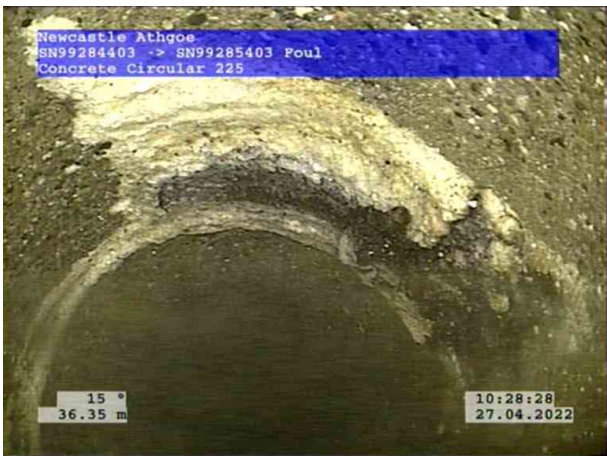
7, 00:04:08, 36.35 m Attached deposits, encrustation at joint from 12 o'clock to 6 o'clock, 10% cross-sectional area loss
