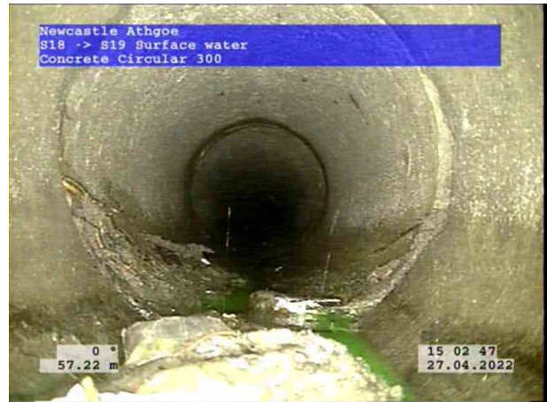
18, 00:05:53, 57.22 m Roots, mass at joint, 15% cross-sectional area loss
