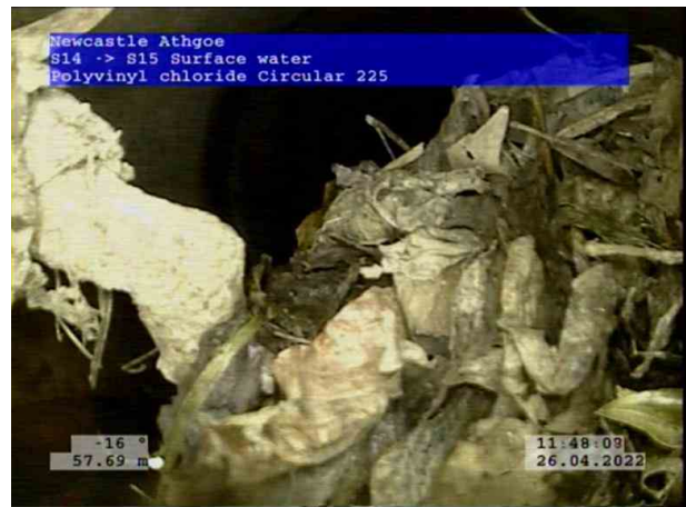
4, 00:05:58, 57.69 m Survey abandoned, NEEDS JETTING
