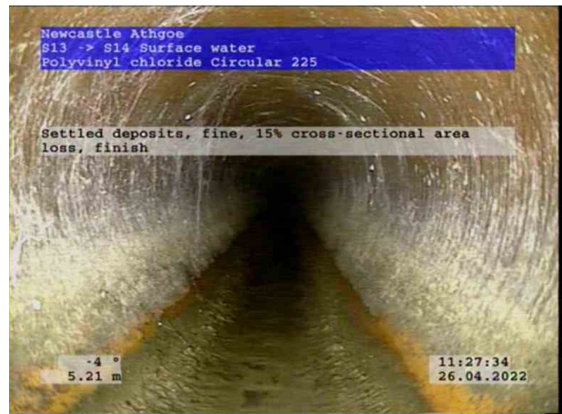
4, 00:04:11, 5.21 m Settled deposits, fine, 15% cross-sectional area loss, finish
