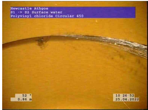
2, 00:00:16, 0.86 m Open joint, large
