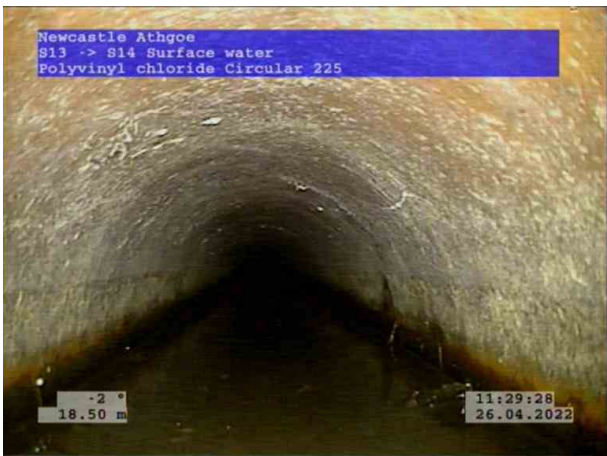
7, 00:05:50, 18.48 m Settled deposits, coarse, 20% cross-sectional area loss
