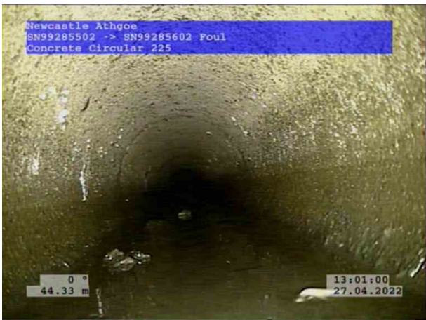
7, 00:04:20, 44.33 m Ingress of gravel from 5 o'clock to 7 o'clock, 10% cross-sectional area loss, start
