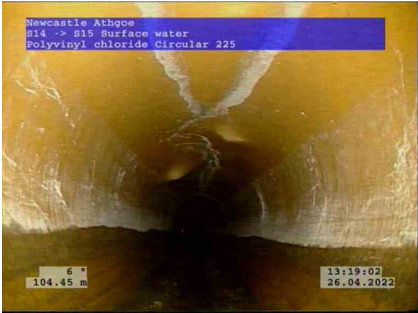
17, 00:13:55, 104.45 m Deformed sewer or drain, 5%
