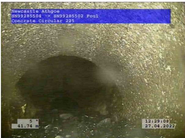
11, 00:04:49, 41.74 m Finish node, manhole, reference: SN99285504, MANHOLE FULL OF GRAVEL
