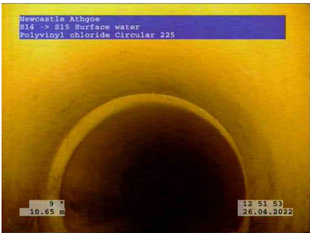
3, 00:00:58, 10.65 m Joint displaced, medium
