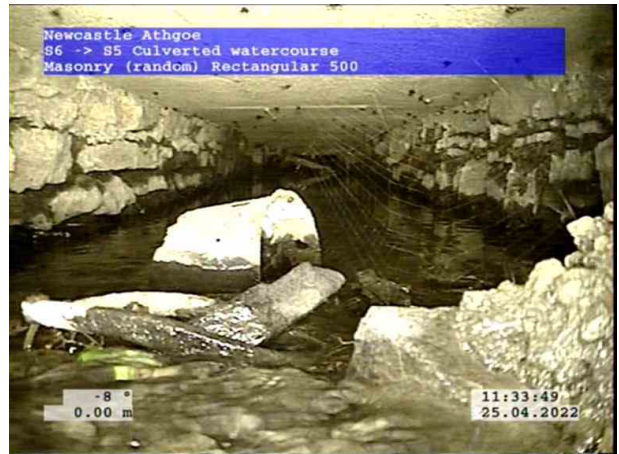
2, 00:00:06, 0.00 m Ingress of gravel from 4 o'clock to 8 o'clock, 20% cross-sectional area loss
