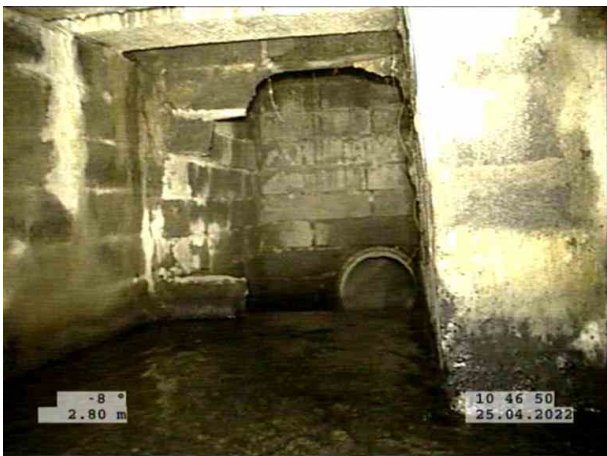
3, 00:00:52, 2.80 m Finish node, other special chamber, reference: S4, HOLDING TANK
