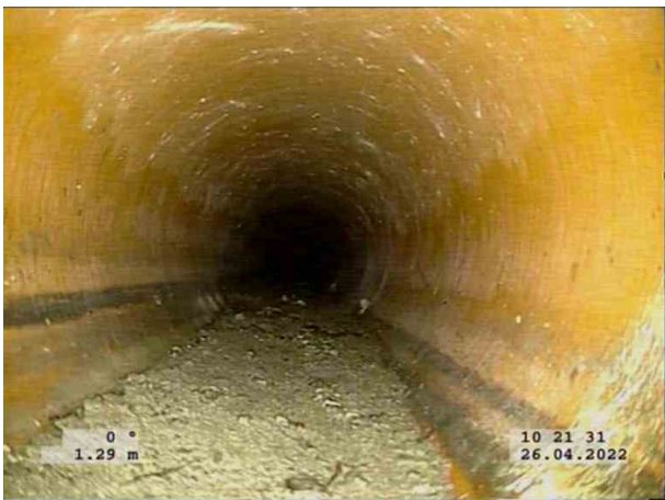
3, 00:00:27, 1.29 m Settled deposits, fine, 10% cross-sectional area loss, start
