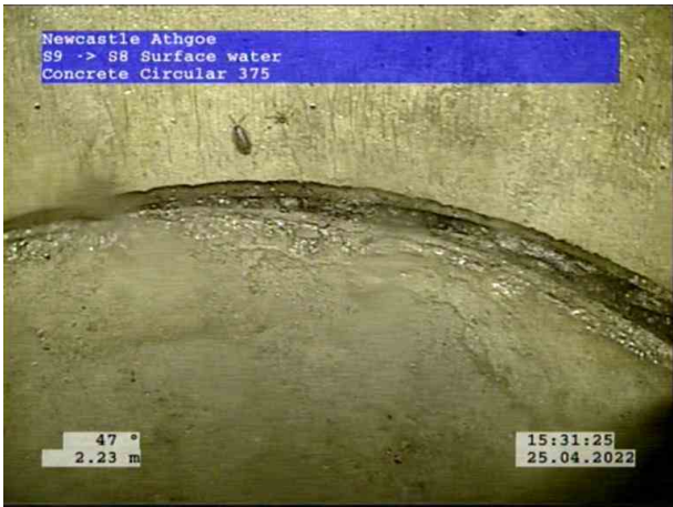
5, 00:00:52, 2.23 m Joint displaced, medium
