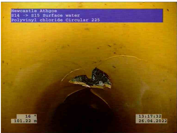
15, 00:12:42, 101.22 m Hole in drain or sewer from 11 o'clock to 1 o'clock
