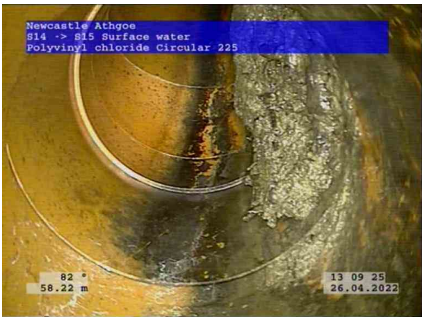
7, 00:05:22, 58.22 m Connection other than junction at 2 o'clock, 225mm dia
