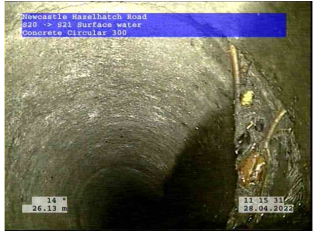
2, 00:01:35, 26.13 m Roots, fine at joint
