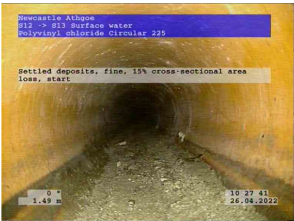
3, 00:00:19, 1.49 m Settled deposits, fine, 15% cross-sectional area loss, start
