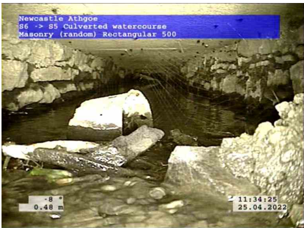
3, 00:00:08, 0.48 m Survey abandoned, ECXTENSIVE JETTING REQUIRED.
