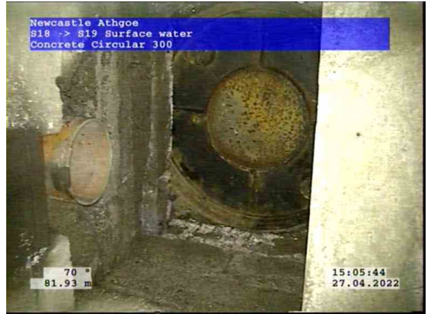
22, 00:08:17, 81.93 m Finish node, manhole, reference: S19, SILT TRAP MANHOLE
