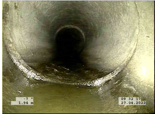
2, 00:00:36, 1.94 m Joint displaced, medium
