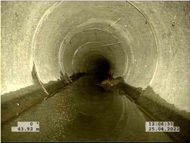
13, 00:06:25, 43.92 m Settled deposits, fine, 10% cross-sectional area loss, start
