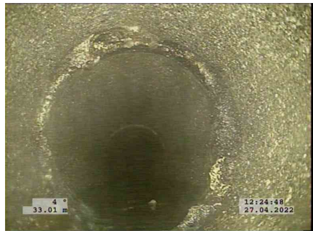
4, 00:03:10, 33.01 m Attached deposits, encrustation at joint from 12 o'clock to 12 o'clock, 10% cross-sectional area loss
