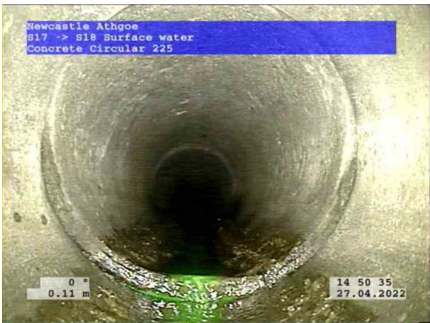
3, 00:00:09, 0.11 m Joint displaced, medium, start
