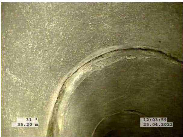
7, 00:04:33, 35.20 m Joint displaced, medium, start
