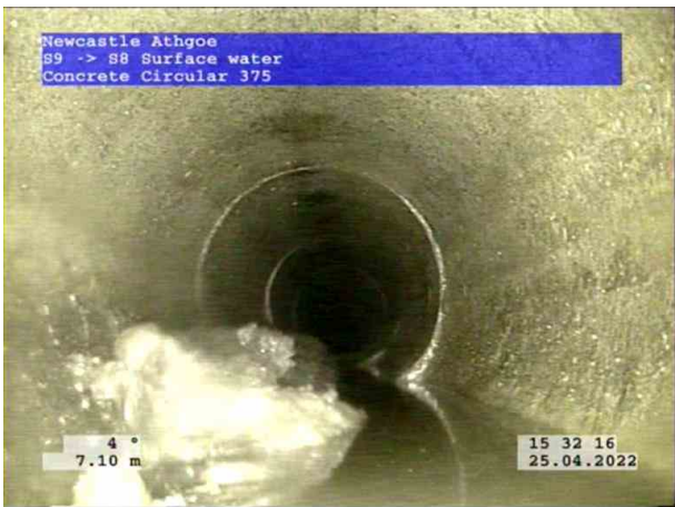
7, 00:01:29, 7.10 m Settled deposits, fine, 15% cross-sectional area loss
