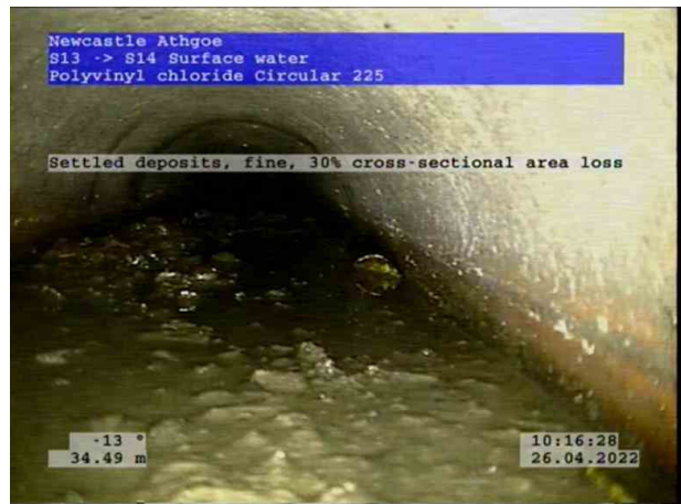
4, 00:02:36, 34.49 m Settled deposits, fine, 30% cross-sectional area loss
