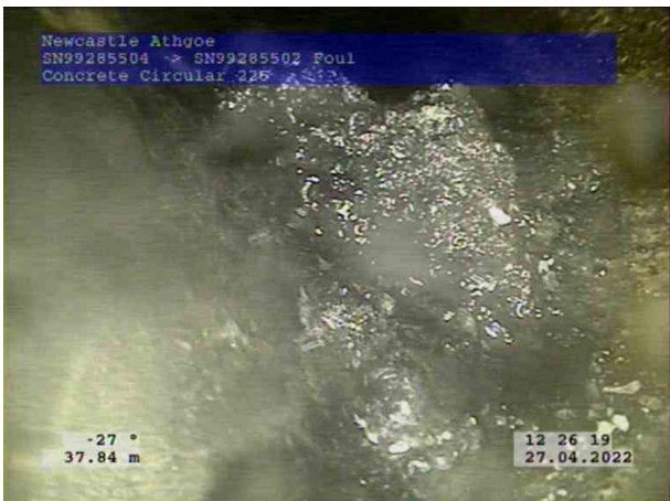
7, 00:04:06, 37.84 m Settled deposits, hard or compacted, 15% cross-sectional area loss
