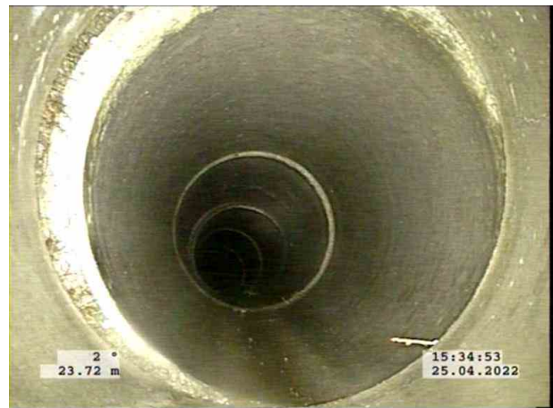
16, 00:03:27, 23.72 m Joint displaced, large
