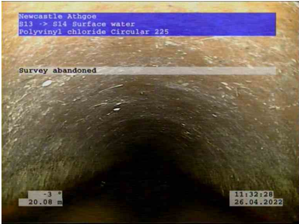
9, 00:08:22, 20.08 m Survey abandoned, UNABLE TO SURVEY. EXTENSIVE JETTING REQUIRED
