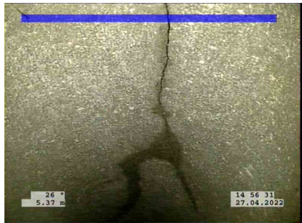
4, 00:00:34, 5.37 m Fracture, longitudinal at 12 o'clock
