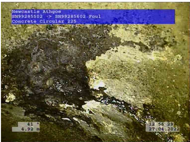
3, 00:00:47, 4.92 m Attached deposits, encrustation at joint from 12 o'clock to 12 o'clock, 5% cross-sectional area loss
