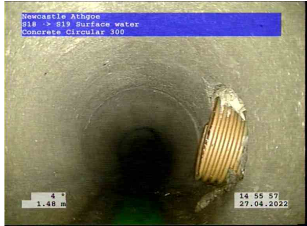
2, 00:00:11, 1.48 m Connection defective, connecting pipe is intruding at 3 o'clock, 150mm dia, intrusion: 5%
