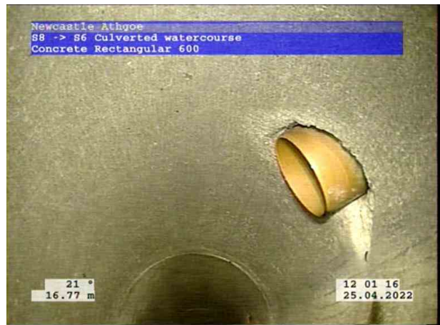
4, 00:02:03, 16.77 m Connection defective, connecting pipe is intruding at 1 o'clock, 100mm dia, intrusion: 5%
