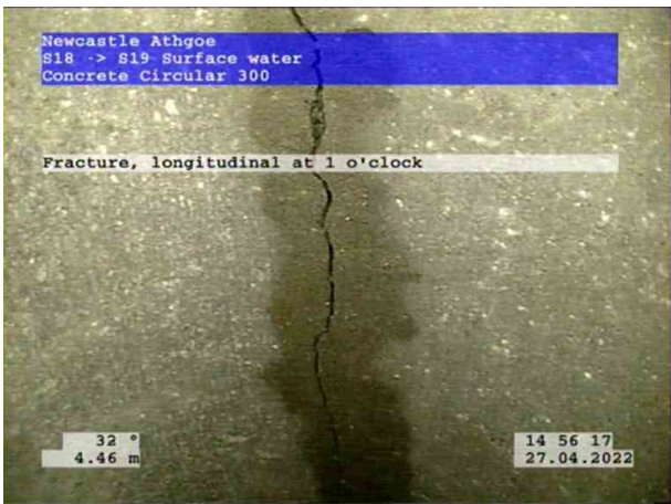
3, 00:00:25, 4.46 m Fracture, longitudinal at 1 o'clock
