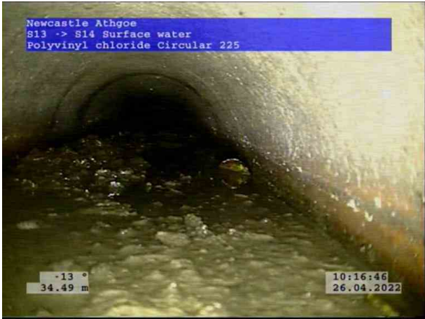
5, 00:02:38, 34.49 m Survey abandoned, UNABLE TO SURVEY. ECXTENSIVE JETTING REQUIRED.
