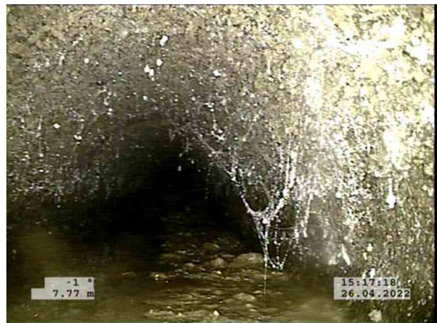
4, 00:01:34, 7.77 m Survey abandoned, unable to survey. jetting required.
