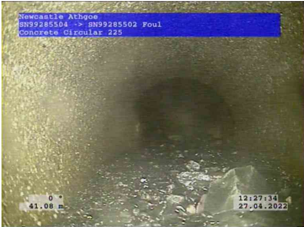
9, 00:04:30, 41.08 m Ingress of gravel from 4 o'clock to 8 o'clock, 30% cross-sectional area loss
