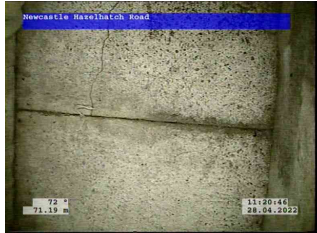
6, 00:06:21, 71.19 m Finish node, manhole, reference: S21, BURIED. NO COVER. GULLY CONNECTED
