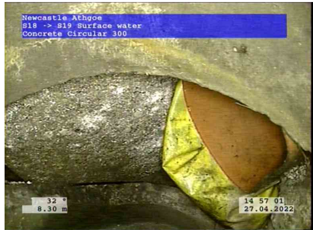
6, 00:00:59, 8.30 m Hole in drain or sewer from 11 o'clock to 1 o'clock
