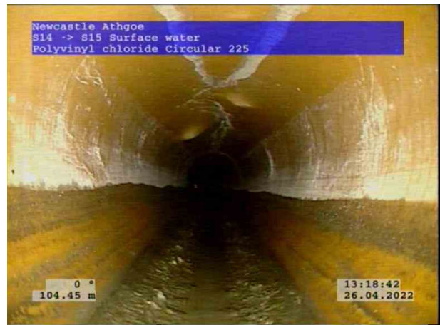
16, 00:13:46, 104.45 m Settled deposits, fine, 5% cross-sectional area loss
