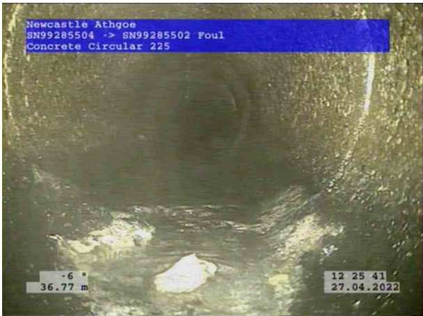
5, 00:03:43, 36.77 m Settled deposits, hard or compacted, 5% cross-sectional area loss
