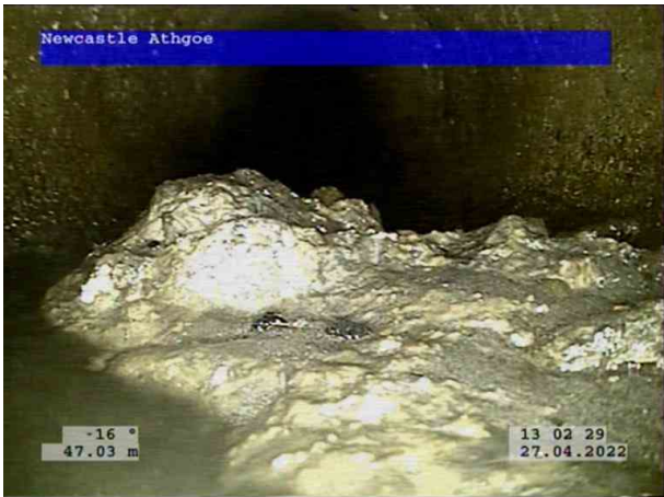
9, 00:05:19, 47.03 m Settled deposits, hard or compacted, 20% cross-sectional area loss
