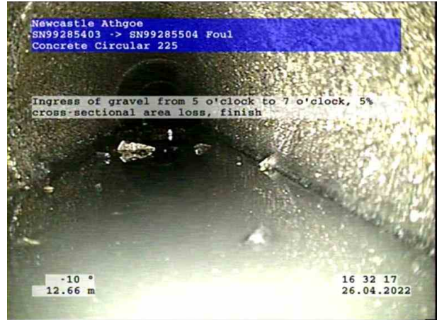
6, 00:02:57, 12.66 m Ingress of gravel from 5 o'clock to 7 o'clock, 5% cross-sectional area loss, finish
