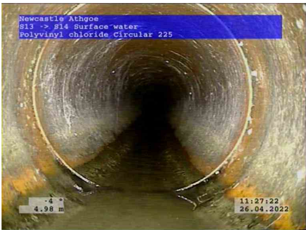
3, 00:04:06, 4.98 m Open joint, large
