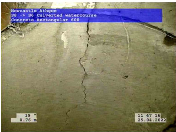
7, 00:01:34, 0.76 m Fracture, longitudinal at 2 o'clock
