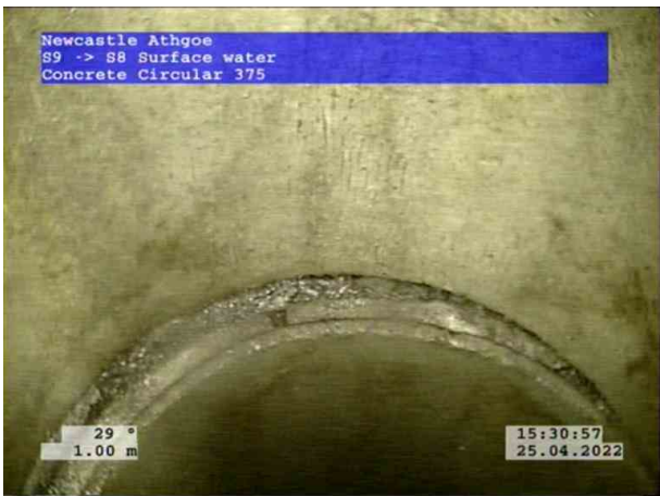
3, 00:00:28, 1.00 m Joint displaced, large
