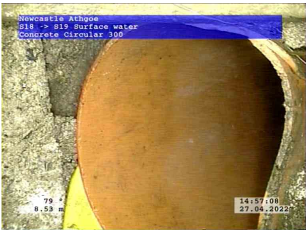
7, 00:01:02, 8.53 m Connection other than junction at 2 o'clock, 150mm dia
