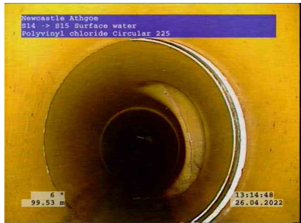
12, 00:10:22, 99.53 m Joint displaced, large
