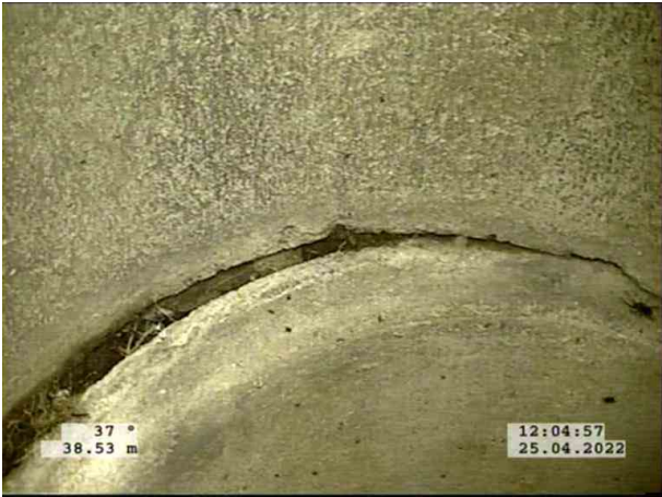
9, 00:05:16, 38.53 m Joint displaced, large
