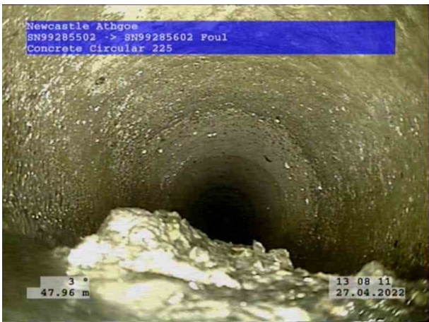
11, 00:05:42, 47.96 m Survey abandoned, settled deposits. cutting required
