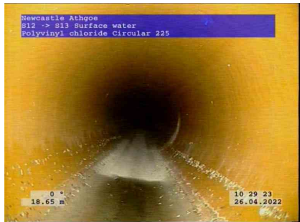
4, 00:01:58, 18.65 m Settled deposits, fine, 15% cross-sectional area loss, finish
