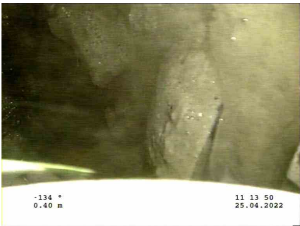
3, 00:00:46, 0.40 m Survey abandoned, SILT IN LINE. ECXTENSIVE JETTING REQUIRED.
