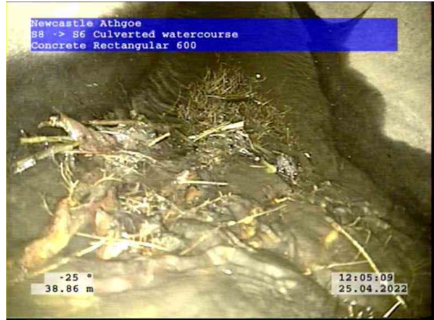
10, 00:05:24, 38.86 m Roots, fine at joint
