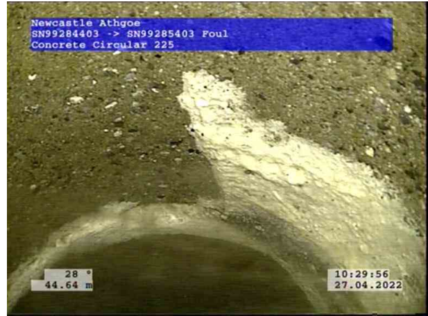
10, 00:05:08, 44.64 m Attached deposits, encrustation from 10 o'clock to 5 o'clock, 5% cross-sectional area loss
