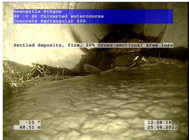
16, 00:07:38, 48.51 m Settled deposits, fine, 20% cross-sectional area loss
