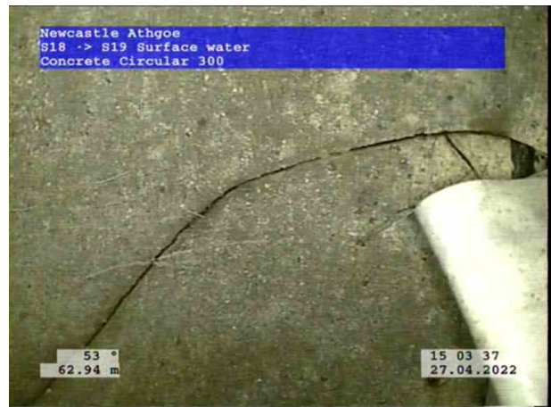
20, 00:06:28, 62.94 m Fracture, circumferential from 12 o'clock to 12 o'clock
