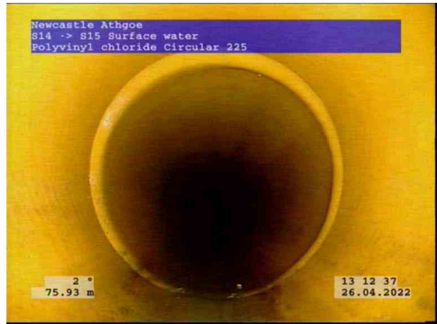
10, 00:08:17, 75.93 m Joint displaced, medium
