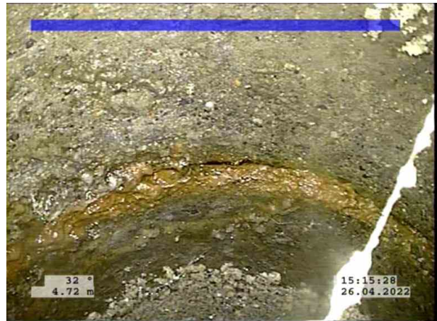
2, 00:00:57, 4.72 m Attached deposits, encrustation at joint from 12 o'clock to 12 o'clock, 5% cross-sectional area loss
