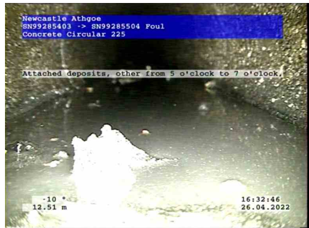
4, 00:03:04, 12.51 m Attached deposits, other from 5 o'clock to 7 o'clock, 15% cross-sectional area loss, stones.
