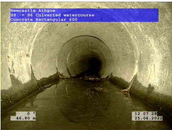
15, 00:07:01, 46.80 m Settled deposits, fine, 15% cross-sectional area loss
