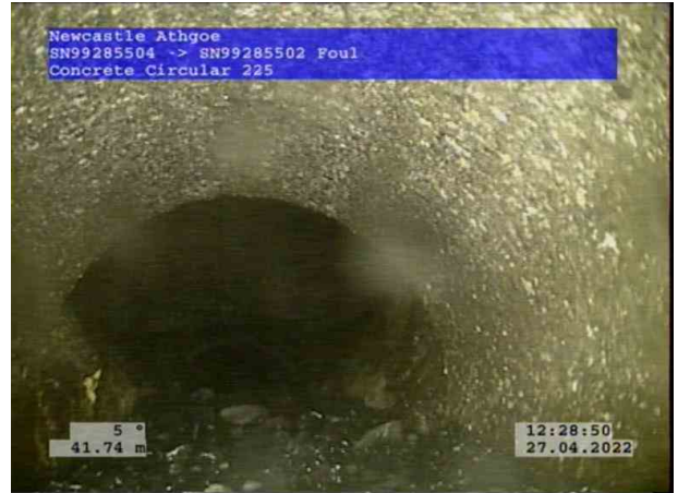
10, 00:04:30, 41.08 m Ingress of gravel from 4 o'clock to 8 o'clock, 30% cross-sectional area loss
