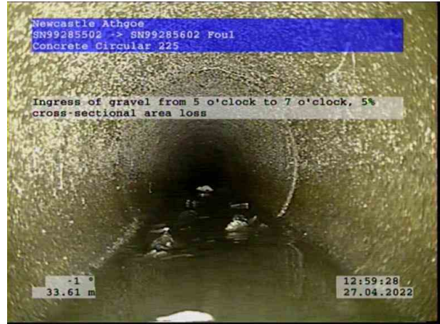
6, 00:03:11, 33.61 m Ingress of gravel from 5 o'clock to 7 o'clock, 5% cross-sectional area loss
