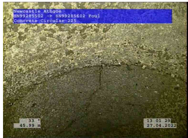
8, 00:04:45, 45.99 m Crack, circumferential from 9 o'clock to 12 o'clock
