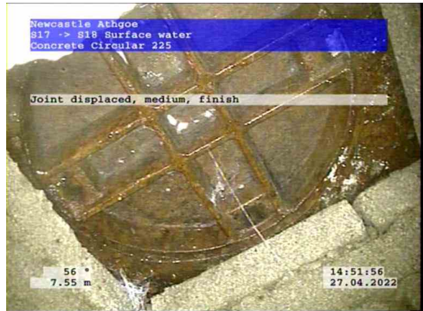
6, 00:01:12, 7.55 m Joint displaced, medium, finish
