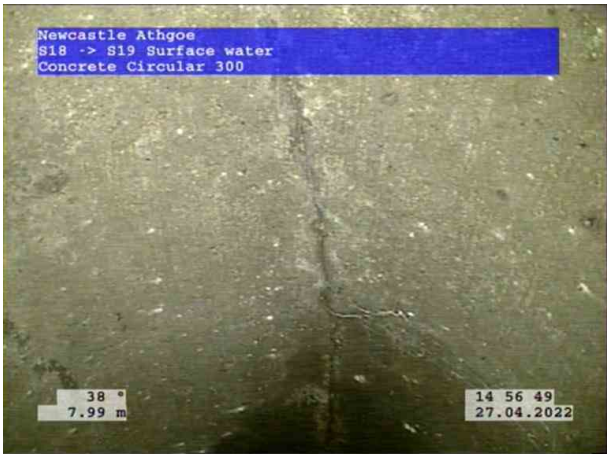
5, 00:00:50, 7.99 m Crack, longitudinal at 12 o'clock
