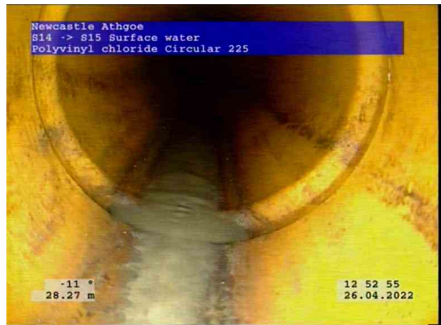
4, 00:01:59, 28.27 m Joint displaced, medium
