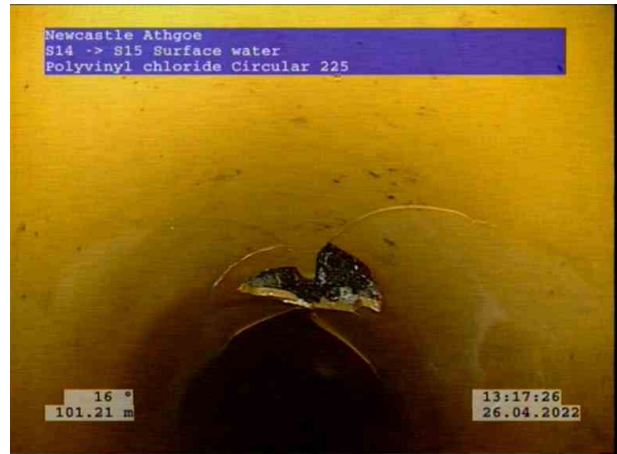
14, 00:12:40, 101.21 m Fractures, multiple from 9 o'clock to 3 o'clock
