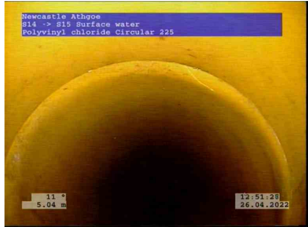
2, 00:00:33, 5.04 m Joint displaced, medium
