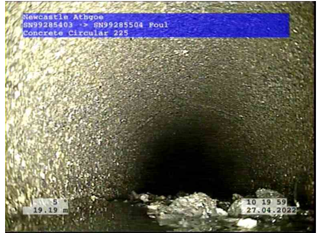
6, 00:02:42, 19.19 m Survey abandoned, GRAVEL IN LINE. ECXTENSIVE JETTING REQUIRED
