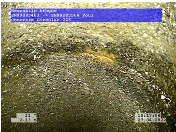
3, 00:00:27, 2.13 m Attached deposits, encrustation at joint from 11 o'clock to 2 o'clock, 5% cross-sectional area loss
