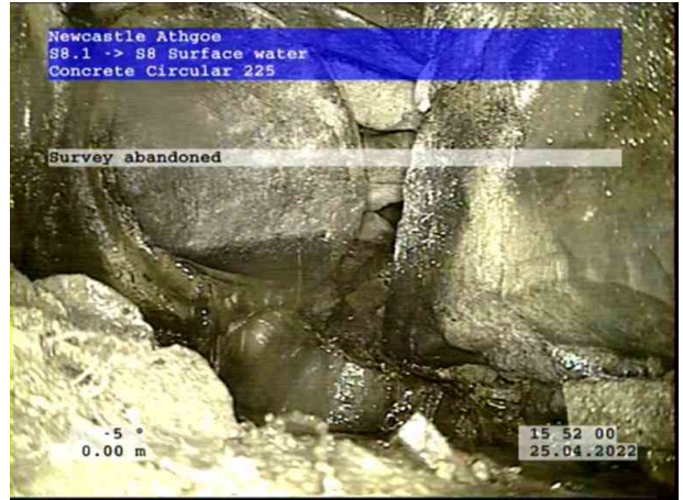
2, 00:00:16, 0.00 m Survey abandoned, UNABLE TO REACH THE PIPE FROM THE MANHOLE.
