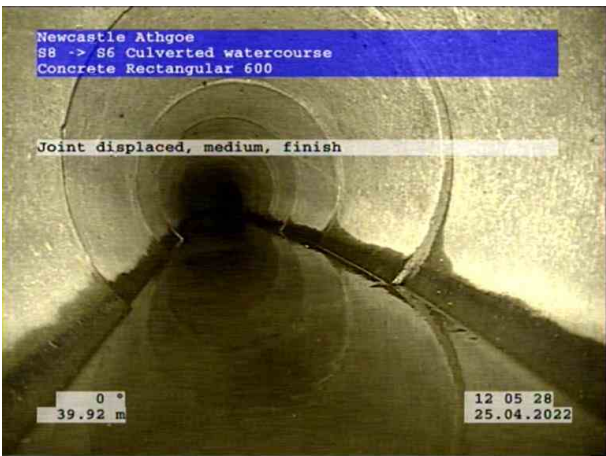
11, 00:05:35, 39.92 m Joint displaced, medium, finish
