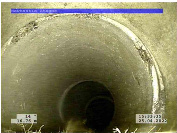
11, 00:02:28, 16.76 m Joint displaced, large
