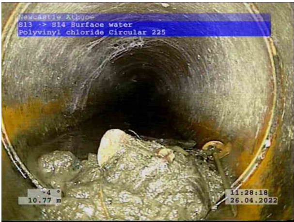
5, 00:04:51, 10.77 m Settled deposits, fine, 20% cross-sectional area loss
