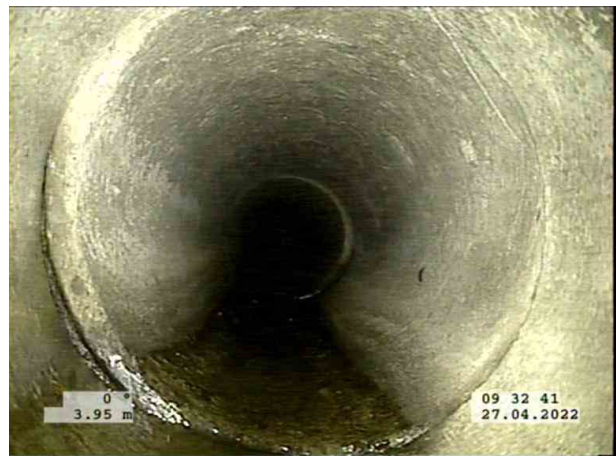
4, 00:00:53, 3.95 m Joint displaced, medium, start
