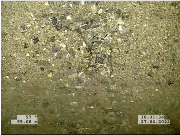
13, 00:06:26, 55.08 m Crack, longitudinal at 1 o'clock
