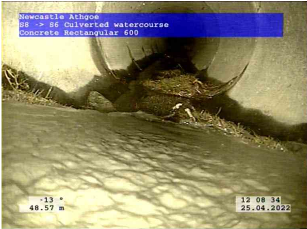
17, 00:07:43, 48.57 m Roots, mass at joint, 20% cross-sectional area loss
