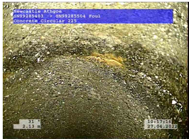
4, 00:00:29, 2.13 m Infiltration, seeping at 1 o'clock
