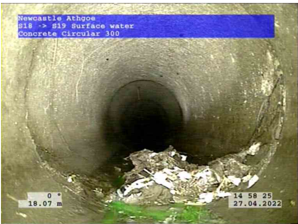
11, 00:02:03, 18.07 m Roots, mass at joint, 10% cross-sectional area loss
