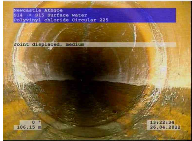
18, 00:15:58, 106.15 m Joint displaced, medium
