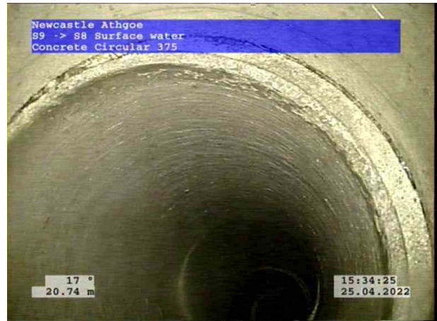
14, 00:03:04, 20.74 m Joint displaced, large
