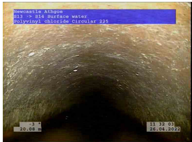
8, 00:08:21, 20.08 m Settled deposits, fine, 10% cross-sectional area loss, finish
