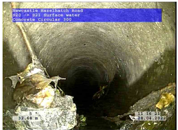
4, 00:02:13, 32.68 m Roots, mass at joint, 15% cross-sectional area loss
