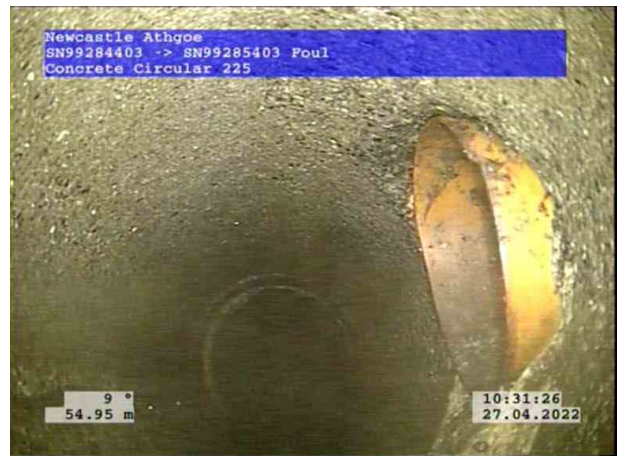
12, 00:06:19, 54.95 m Connection defective, connecting pipe is intruding at 3 o'clock, 150mm dia, intrusion: 5%
