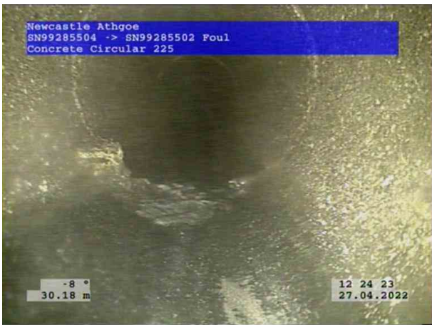
3, 00:02:55, 30.18 m Attached deposits, encrustation at joint from 5 o'clock to 7 o'clock, 5% cross-sectional area loss
