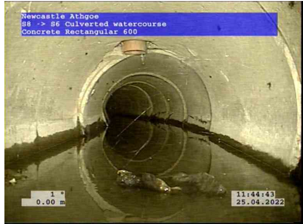
2, 00:00:09, 0.00 m Settled deposits, fine, 10% cross-sectional area loss
