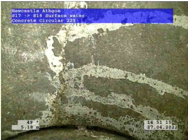
5, 00:00:40, 5.18 m Crack, longitudinal at 1 o'clock
