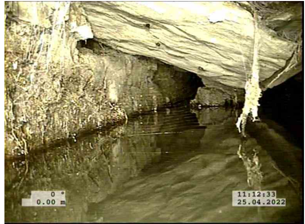
2, 00:00:10, 0.00 m Settled deposits, fine, 20% cross-sectional area loss
