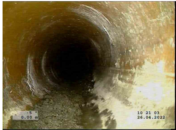
2, 00:00:09, 0.00 m Settled deposits, coarse, 5% cross-sectional area loss
