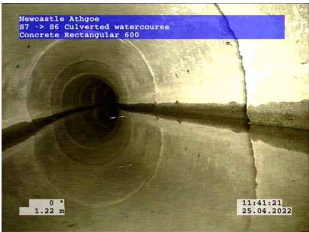
3, 00:01:23, 1.22 m Survey abandoned, ECXTENSIVE JETTING REQUIRED
