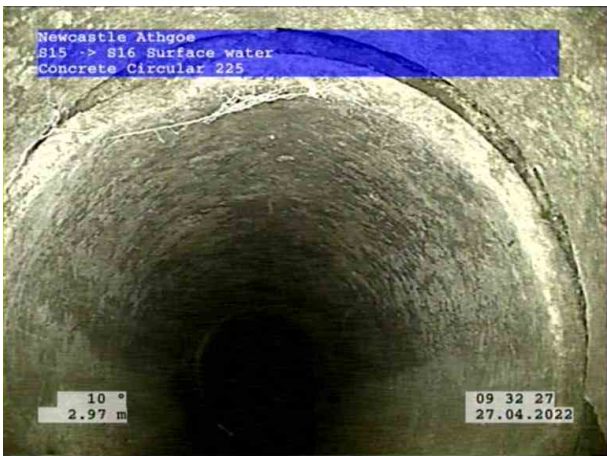
3, 00:00:44, 2.97 m Joint displaced, medium
