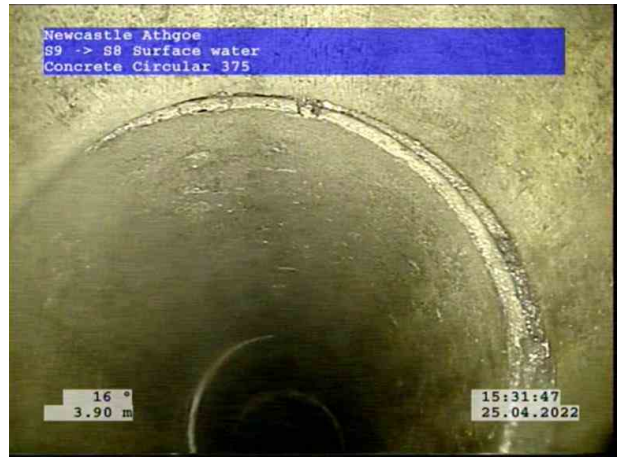
6, 00:01:09, 3.90 m Joint displaced, medium, start
