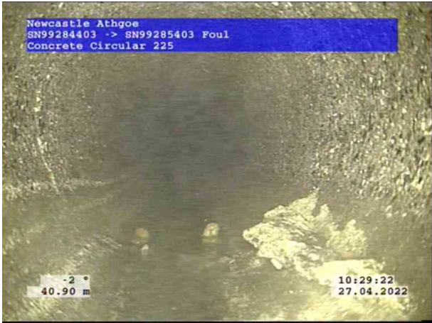
9, 00:04:44, 40.90 m Attached deposits, grease at 4 o'clock, 15% cross-sectional area loss
