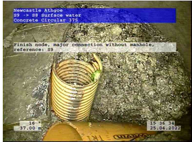
18, 00:04:35, 37.00 m Finish node, major connection without manhole, reference: S9, START OF THE LINE. NO MANHOLE
