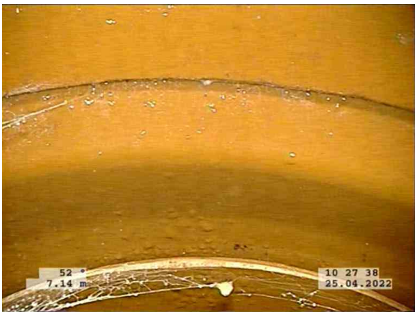
3, 00:00:59, 7.14 m Open joint, large
