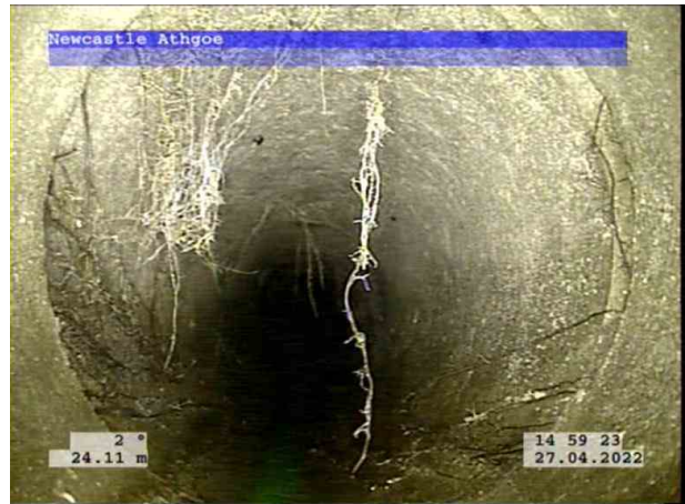
14, 00:02:49, 24.11 m Roots, fine at joint, start
