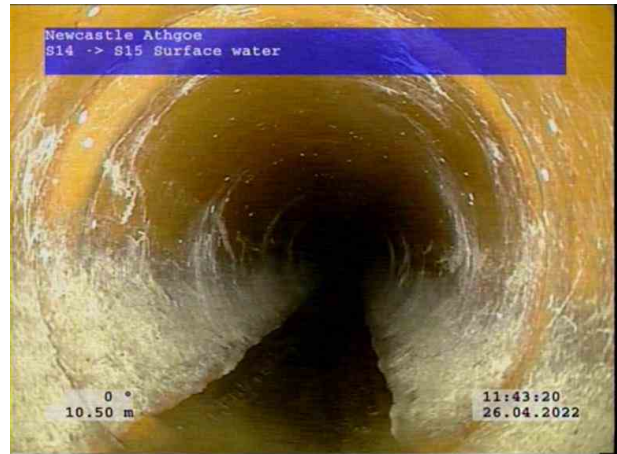
2, 00:01:26, 10.50 m Joint displaced, medium
