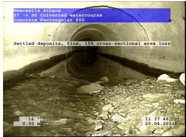
2, 00:00:15, 0.00 m Settled deposits, fine, 15% cross-sectional area loss
