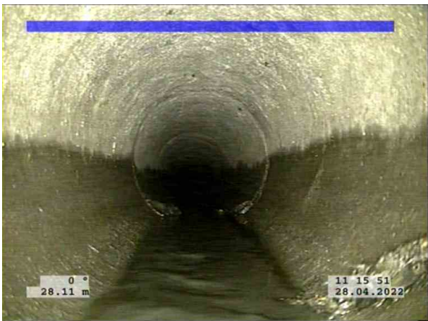
3, 00:01:48, 28.11 m Roots, fine at joint, start
