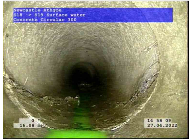
10, 00:01:52, 16.08 m Roots, fine at joint
