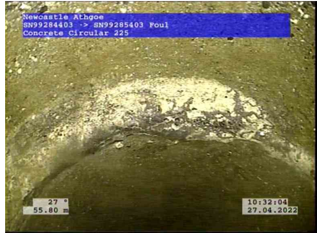
14, 00:06:47, 55.80 m Attached deposits, encrustation from 6 o'clock to 12 o'clock, 10% cross-sectional area loss
