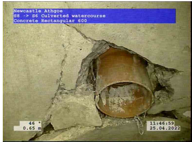
6, 00:01:22, 0.65 m Fractures, multiple from 10 o'clock to 2 o'clock
