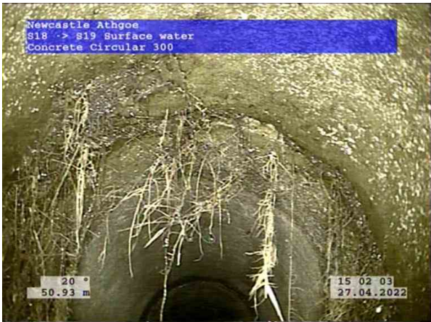
17, 00:05:19, 50.93 m Roots, mass at joint, 10% cross-sectional area loss
