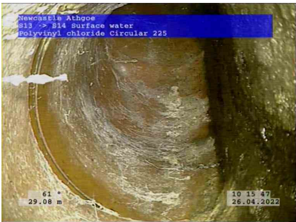
3, 00:02:06, 29.08 m Connection other than junction at 3 o'clock, 150mm dia
