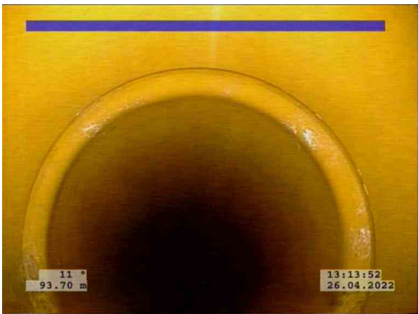
11, 00:09:27, 93.70 m Joint displaced, medium
