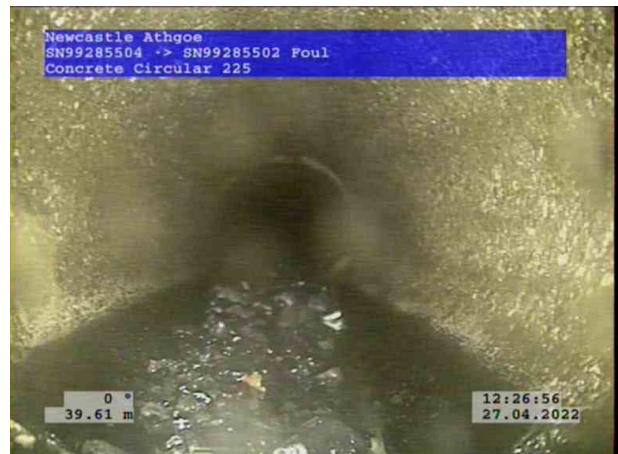
8, 00:04:19, 39.61 m Ingress of gravel from 5 o'clock to 7 o'clock, 10% cross-sectional area loss
