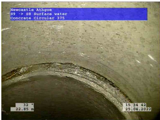
15, 00:03:20, 22.85 m Joint displaced, large
