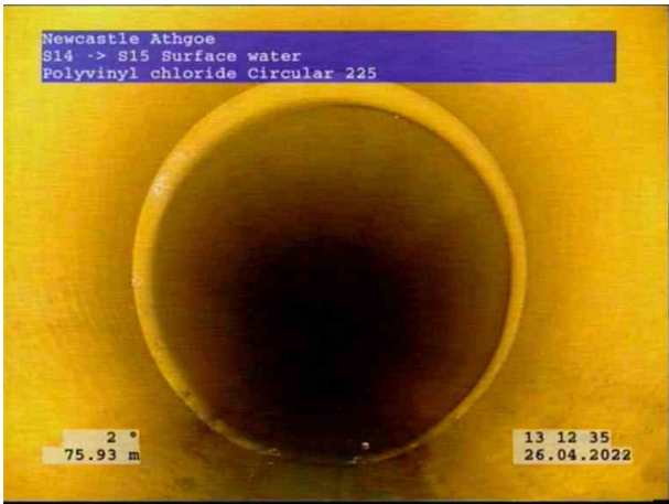
9, 00:05:55, 64.27 m Joint displaced, medium
