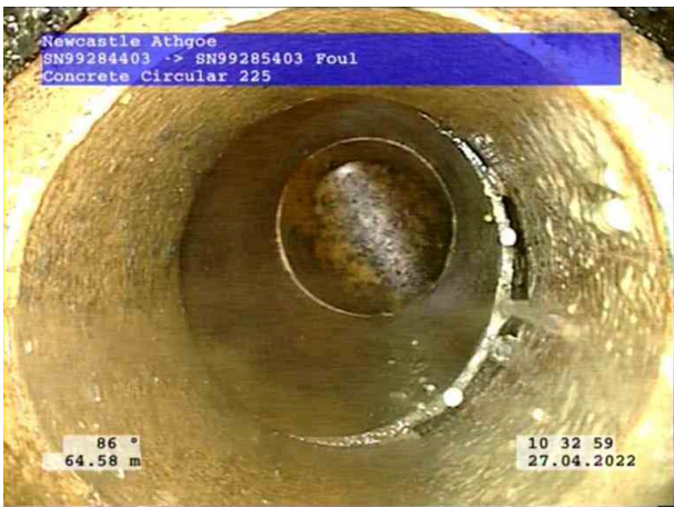
15, 00:07:38, 64.58 m Connection other than junction at 12 o'clock, 100mm dia
