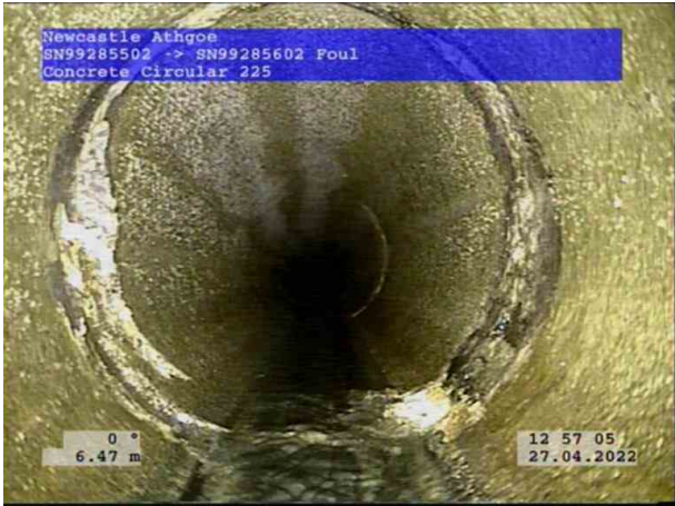
5, 00:01:02, 6.47 m Attached deposits, encrustation at joint from 4 o'clock to 10 o'clock, 5% cross-sectional area loss
