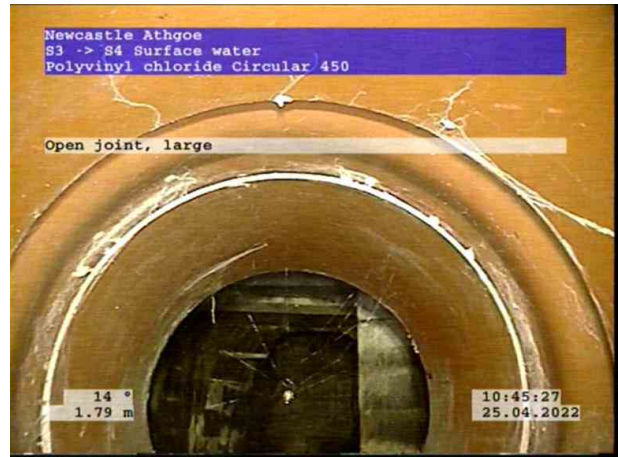
2, 00:00:20, 1.79 m Open joint, large
