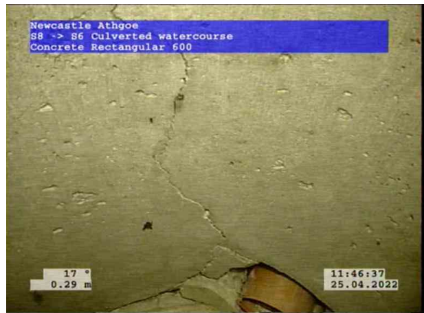
4, 00:01:07, 0.29 m Fracture, longitudinal at 10 o'clock
