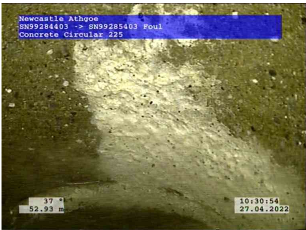
11, 00:05:57, 52.93 m Attached deposits, encrustation from 2 o'clock to 5 o'clock, 5% cross-sectional area loss
