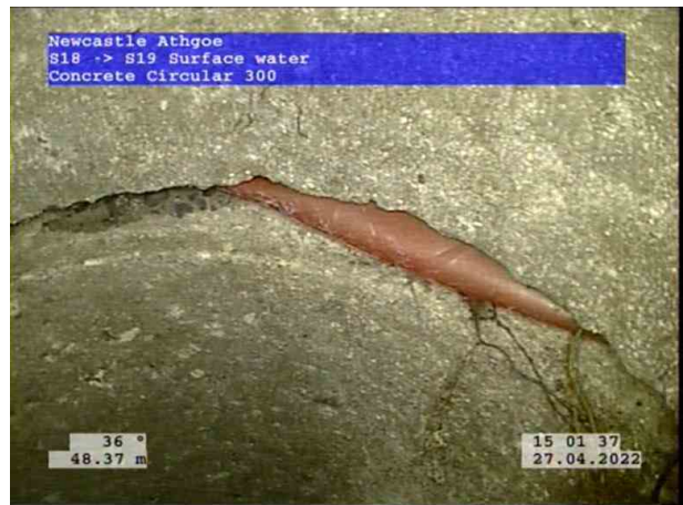
16, 00:05:01, 48.37 m Joint displaced, medium
