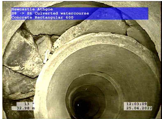
6, 00:03:49, 32.98 m Joint displaced, large
