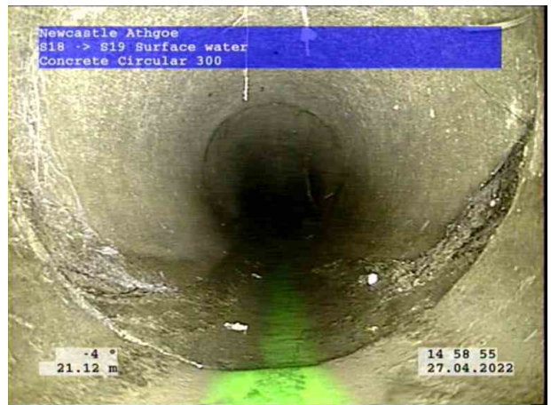
12, 00:02:29, 21.12 m Roots, fine at joint
