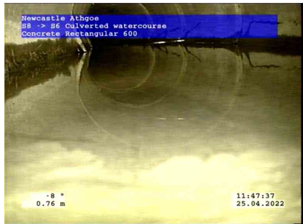
8, 00:01:44, 0.76 m Survey abandoned, SILT IN LINE. ECXTENSIVE JETTING REQUIRED
