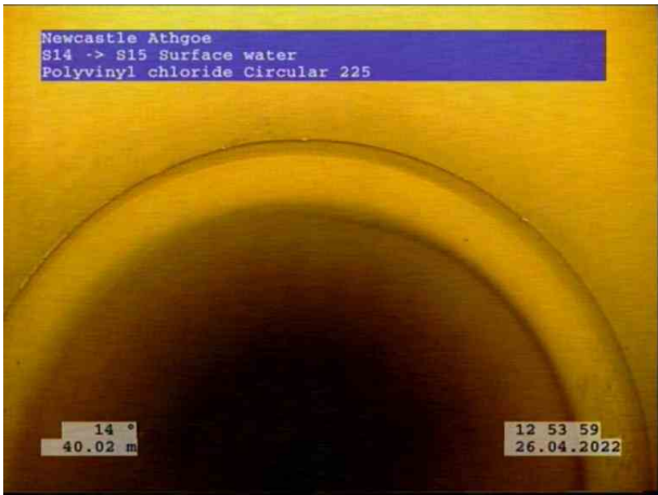
5, 00:03:02, 40.02 m Joint displaced, medium
