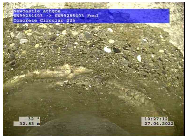
4, 00:03:25, 32.83 m Attached deposits, encrustation from 11 o'clock to 4 o'clock, 5% cross-sectional area loss
