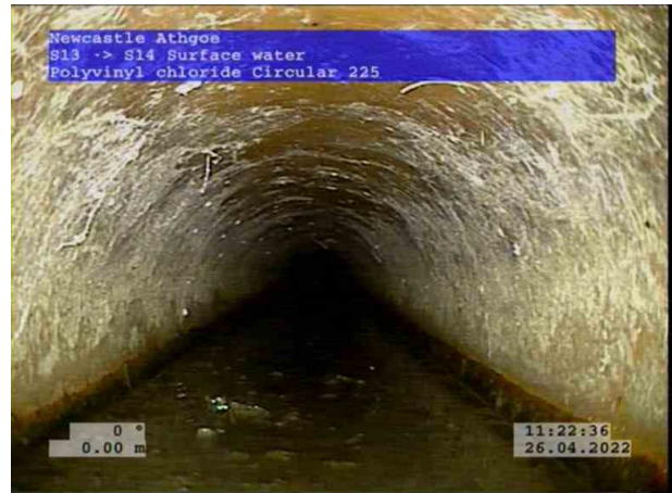
2, 00:00:06, 0.00 m Settled deposits, fine, 15% cross-sectional area loss, start
